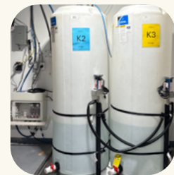
1000L Holding Tanks
